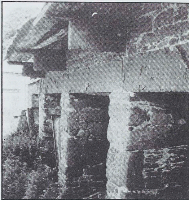
The swept roof over the granary openings, supported on long projecting corbels
