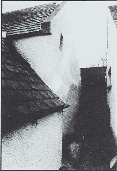
West Elevation : The completed harl which in this case respects rather than hides the sequence
